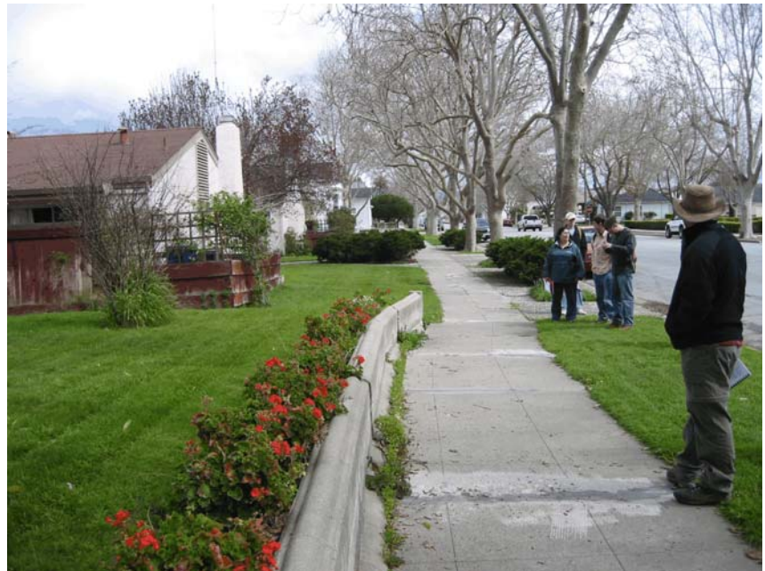
Displaced sidewalk at site F. The three students are standing on the race of the fault.
